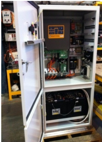
Figure 2: Inside view of an RESS. The inverter and control system are located in the upper compartment and the batteries in the lower compartment.
