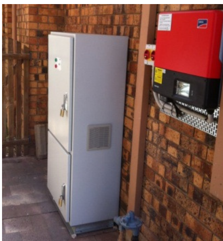
Figure 1: Residential battery storage unit, with solar inverter in foreground
