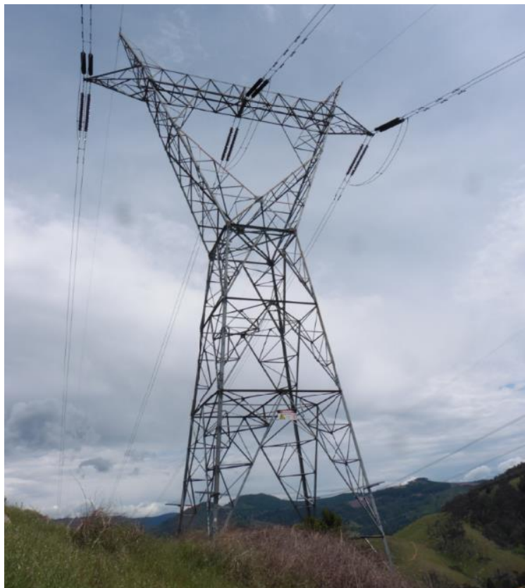
Figure 1: T080 MSS-DDTS No. 2 330 kV strain tower
