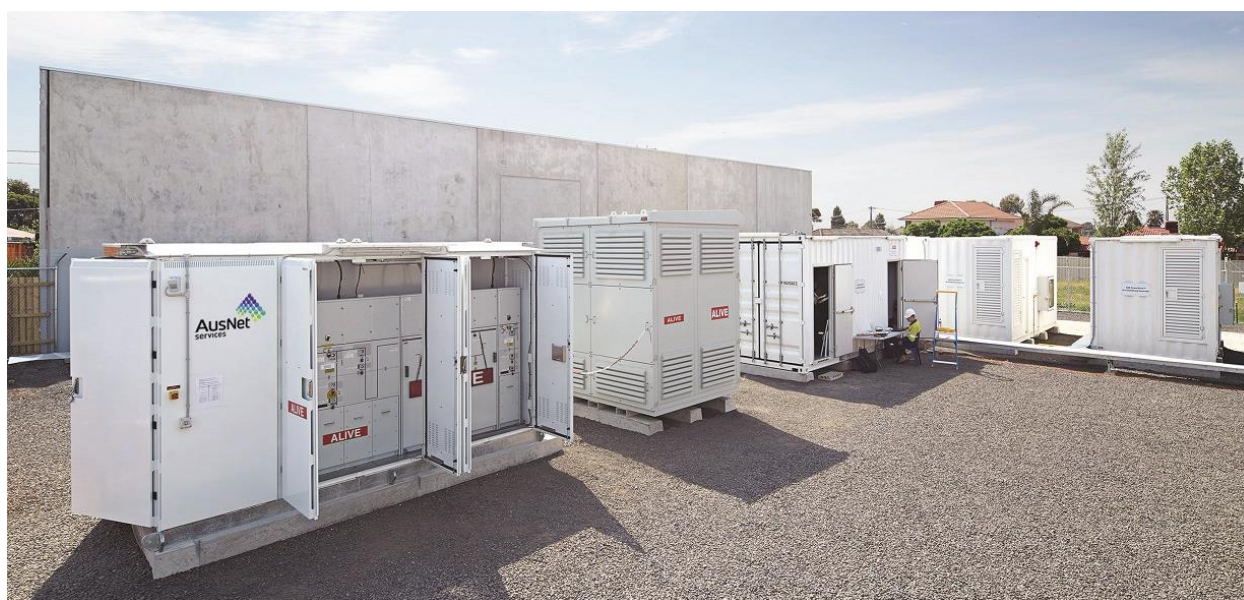
Fig 1: The AusNet Services Grid Energy Storage System, installed in Thomastown (Photo credit: ABB)
