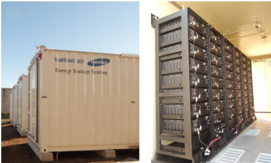
Fig 3 Samsung battery container (left) and battery racks (right)
